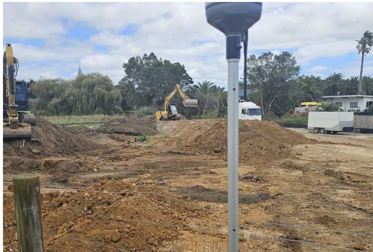
Emlid RS4 base station on site at a residential subdivision, with Cat excavators working in the background
